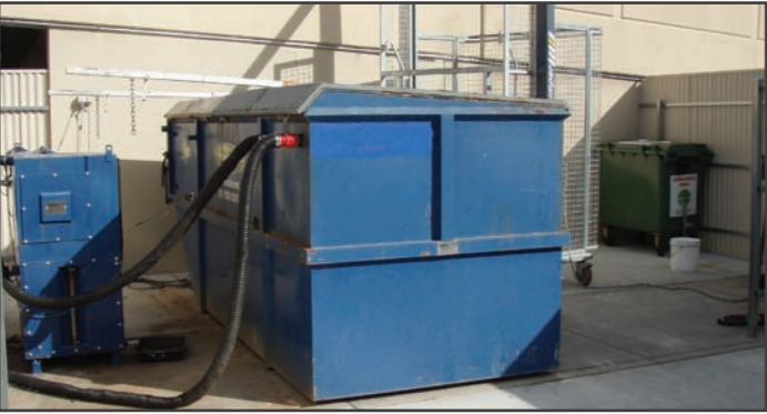
The larger 9m 3 on site capturing organic material from a market place, convention centre & shopping centre.
